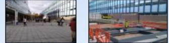
Area between the Hub and James Stanley (building B3) before and during works.
