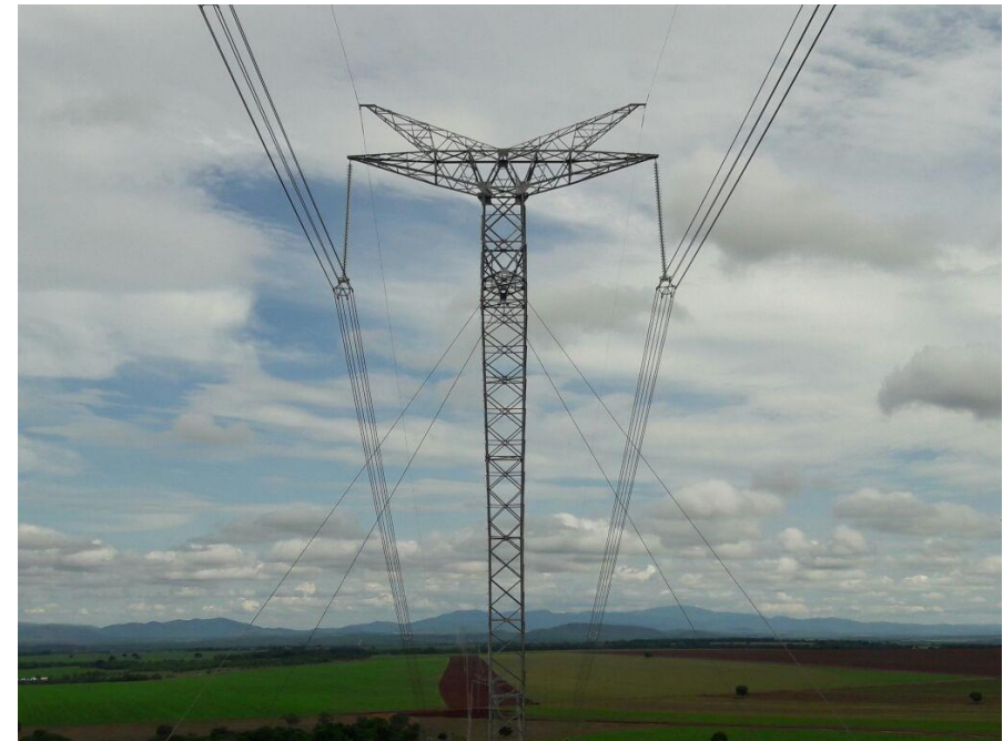
60 kV, Set San Luis - Set Central - Set San Isidro Peru
