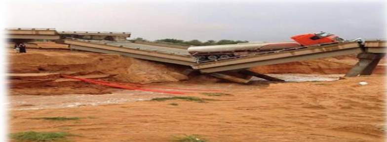
Picture of (scouring at Thumama Wadi bridge)
