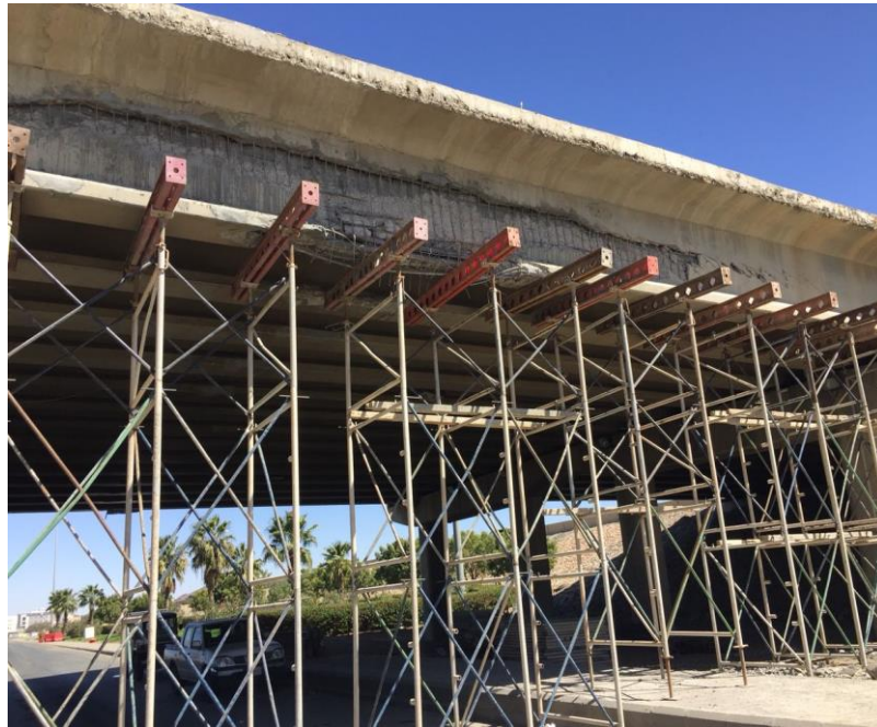
Figure 10.3: Support the damage of girder
