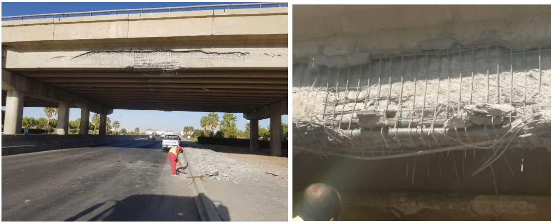
Figure 10.1: Pictures for the damage in the girder
